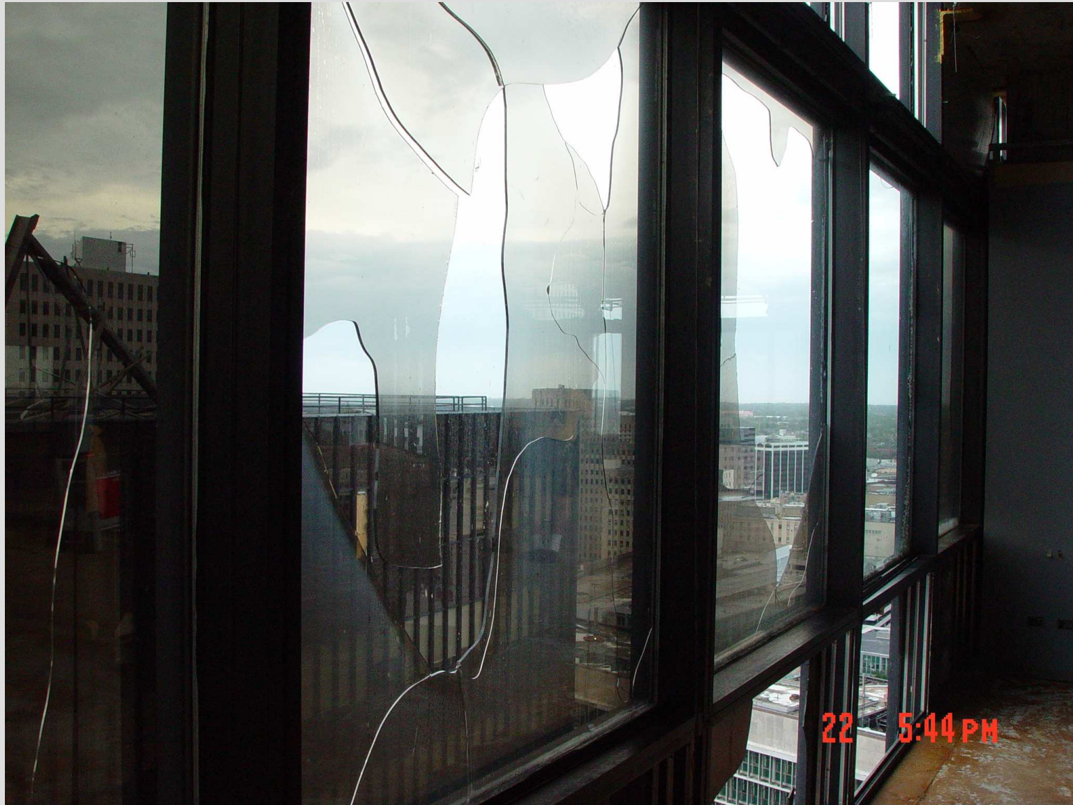
Typical window damage to 1250 Poydras due to wind-borne gravel
