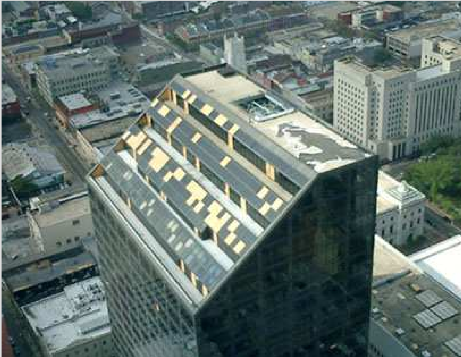
Texaco Building, single-ply ballasted roof, debris source
