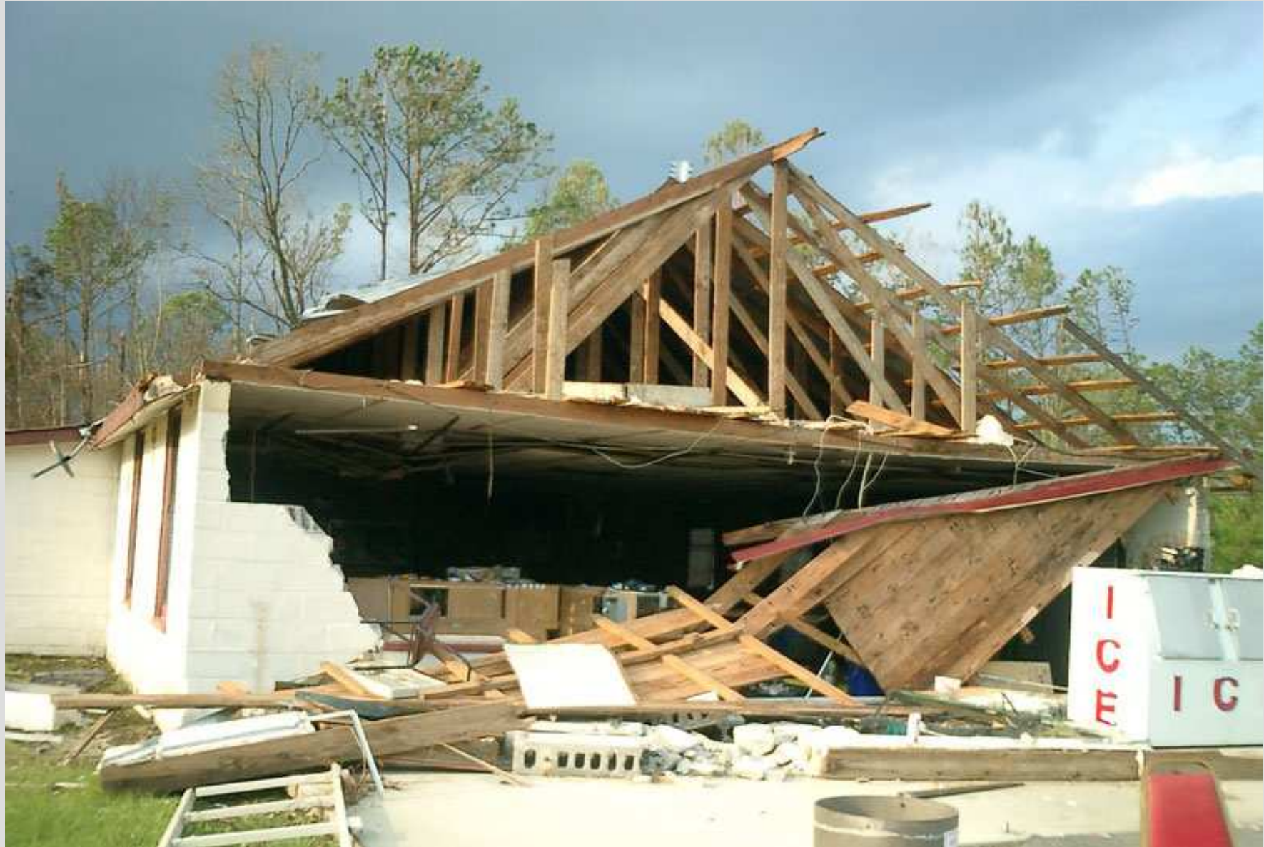
Wind damage to shop structure near Long Beach MS
