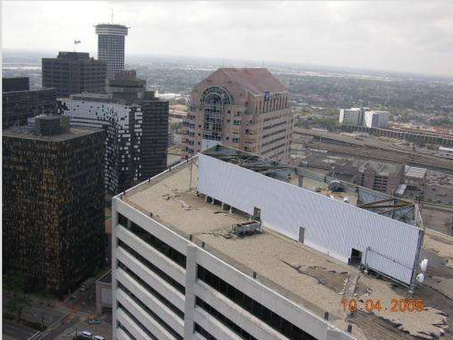
Ballasted single-ply roof - Source of debris causing damage to Amoco and Dominion Bank
