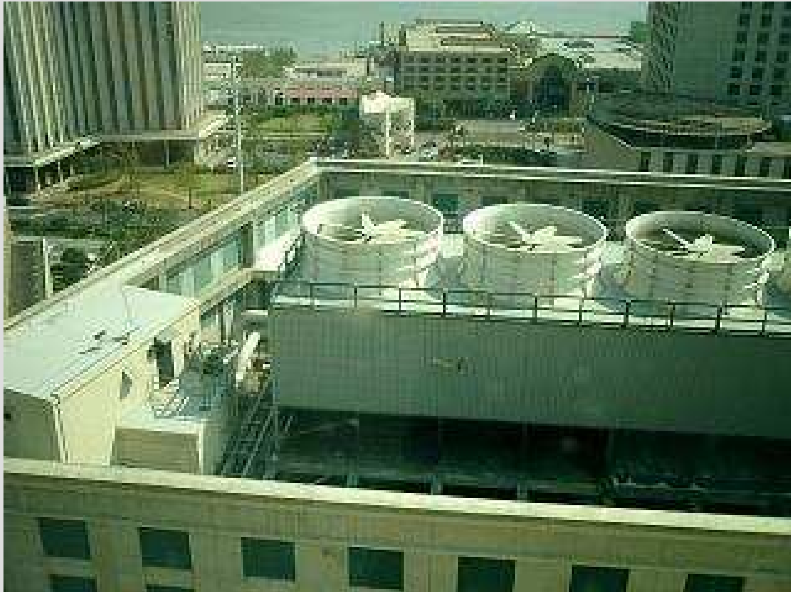
2x4 penetrating cooling tower screen
