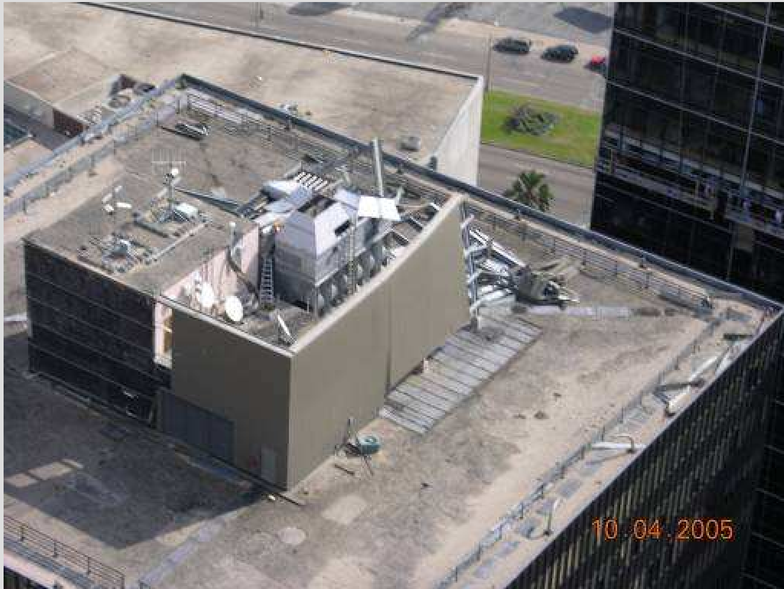
Scoured gravel on Amoco roof, a source of debris causing damage to Hyatt
