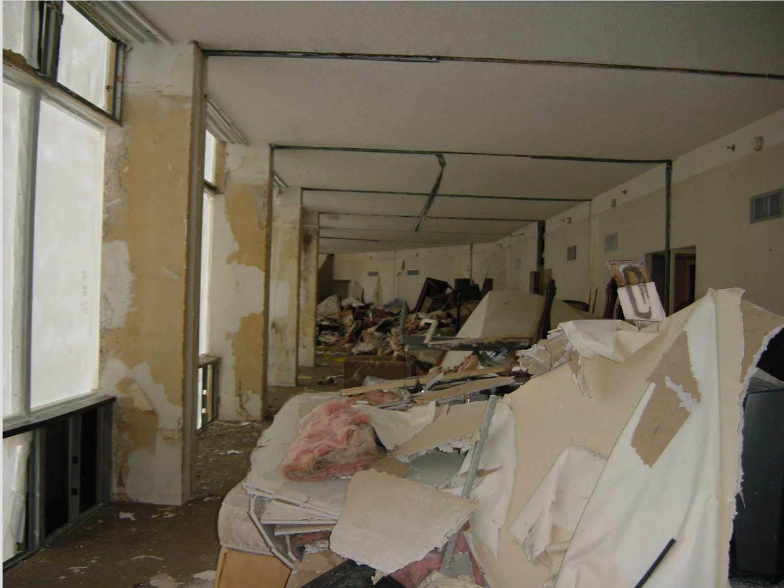
Damage to rooms on north face of 27 th floor
