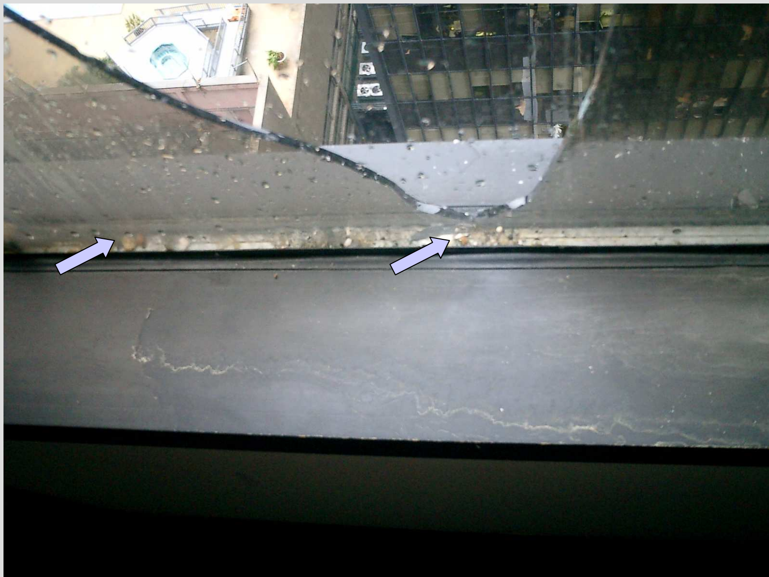
Gravel in the gap between broken outer pane and intact inner pane
