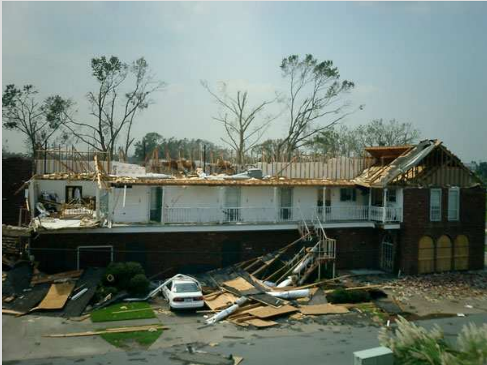
Gable end failure causes loss of roof due to increased internal pressure
