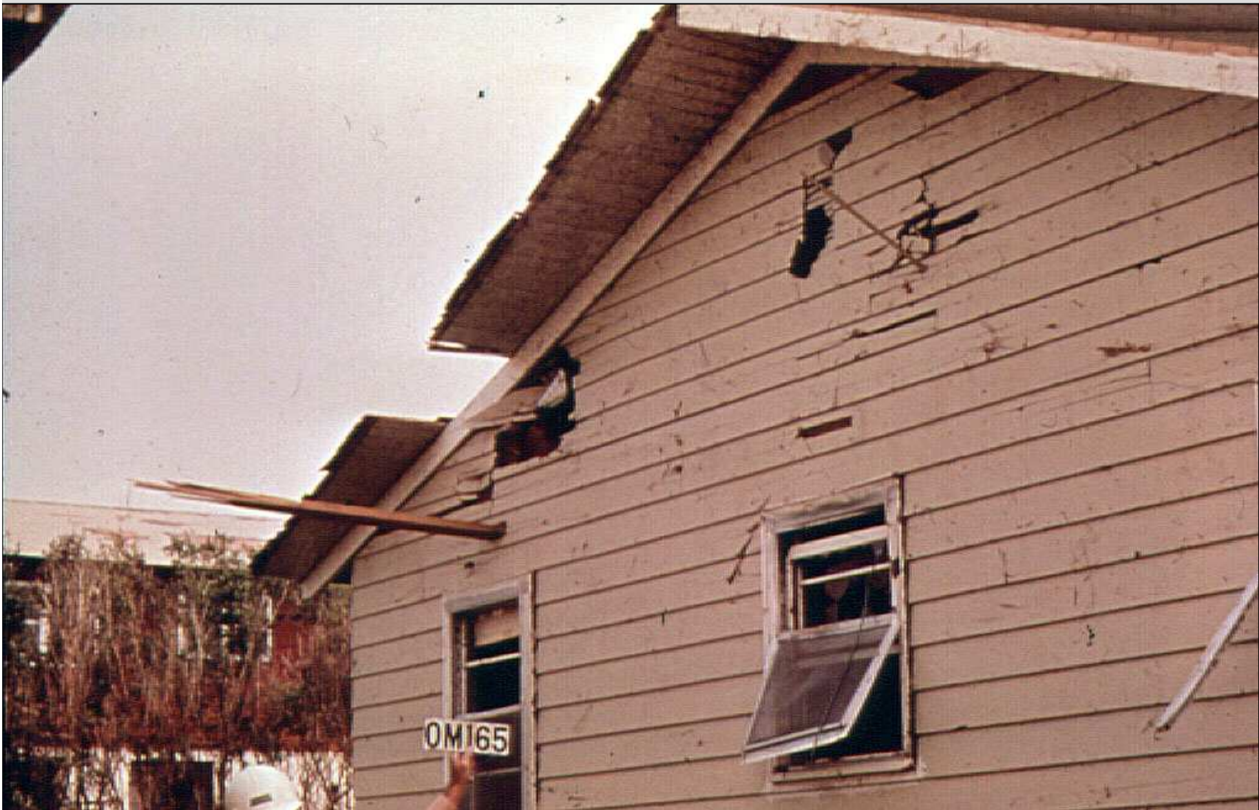
Penetration of wall by flying debris
