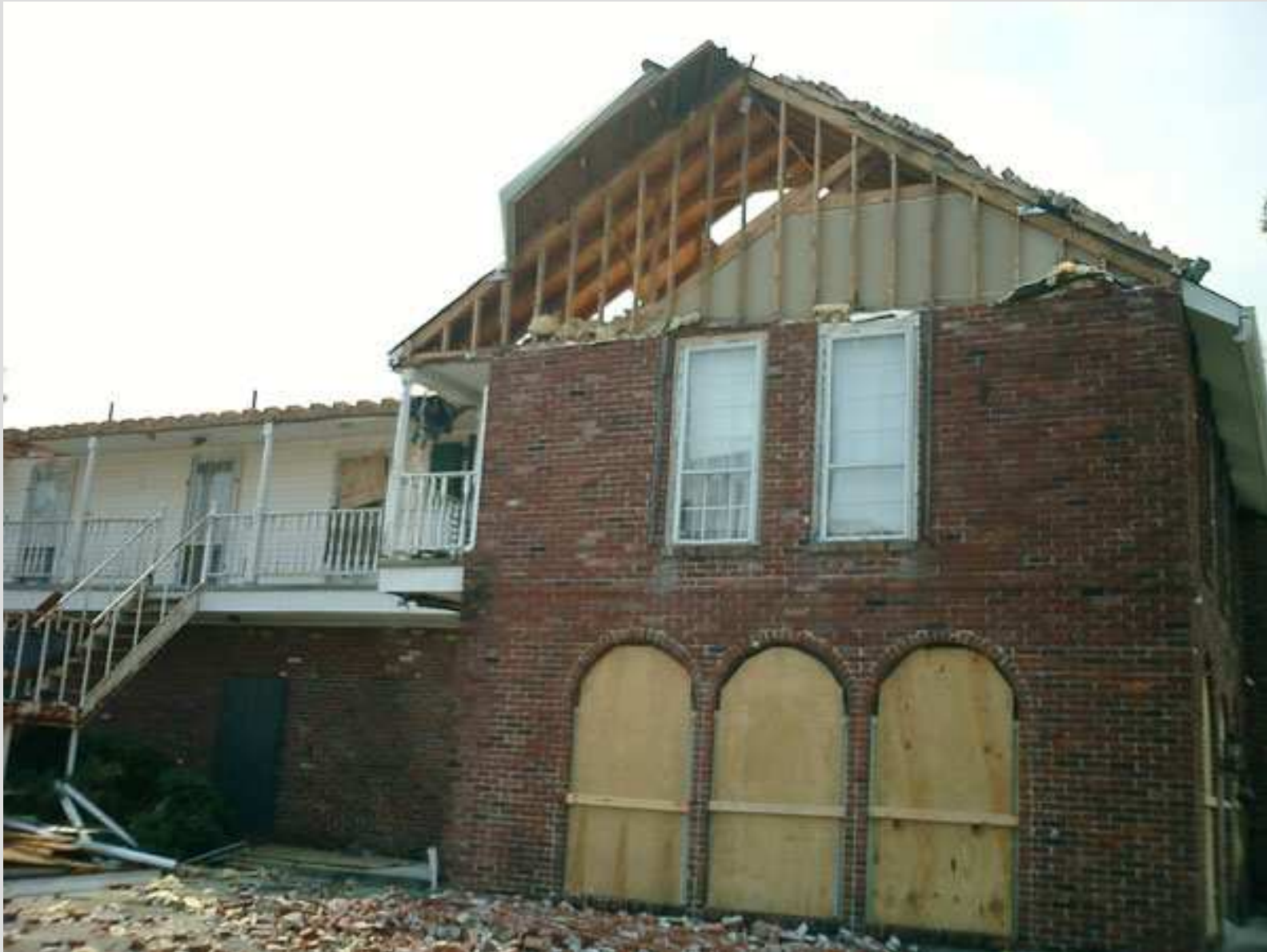
Wind-damaged apartments near West Jefferson Hospital – classic gable end failure
