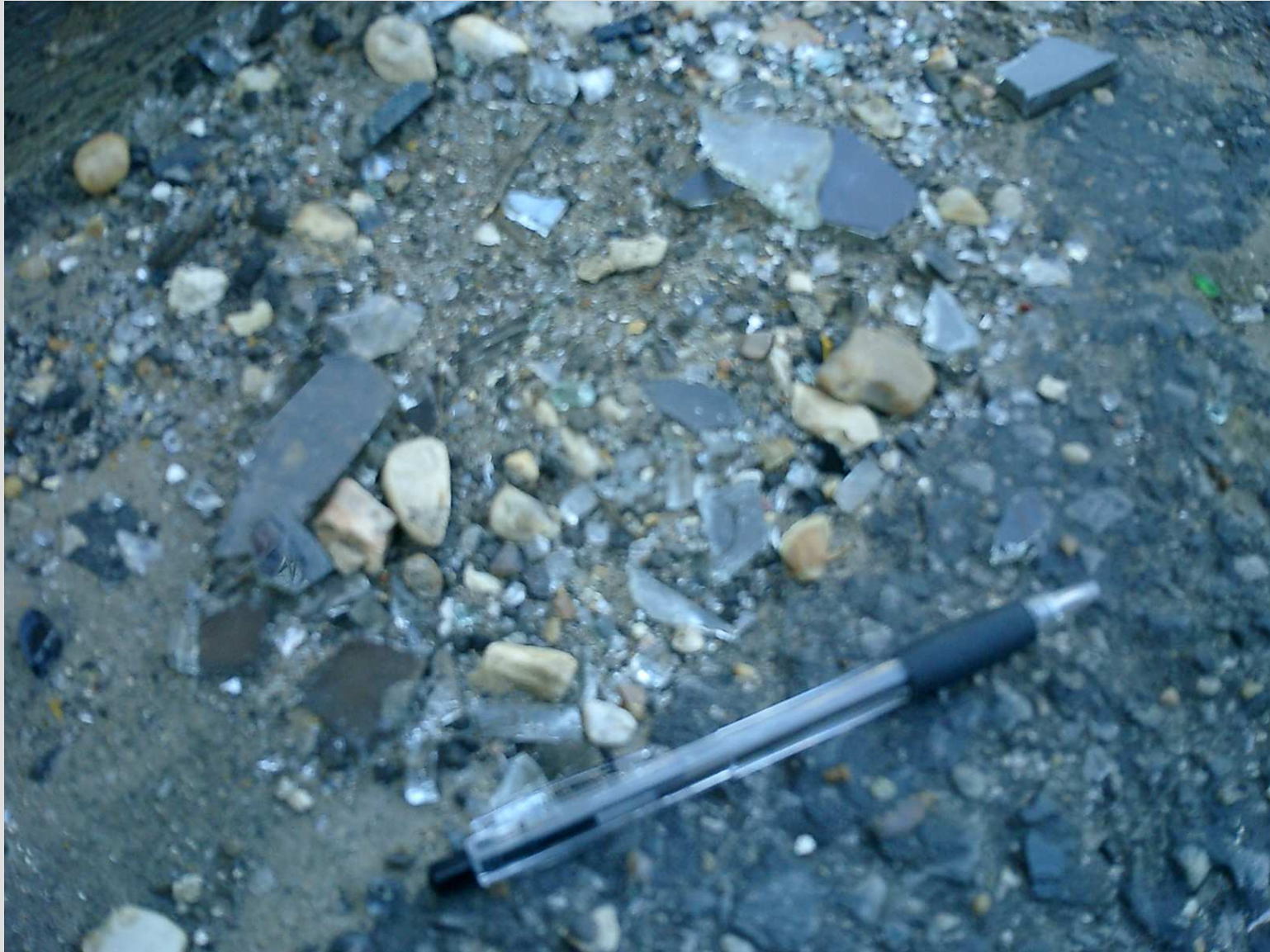
Gravel on sidewalk at base of Amoco
